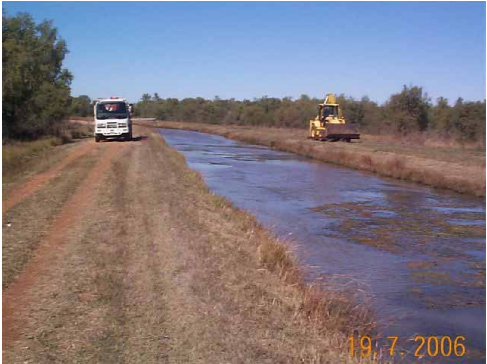
Water Delivery - Open channel
